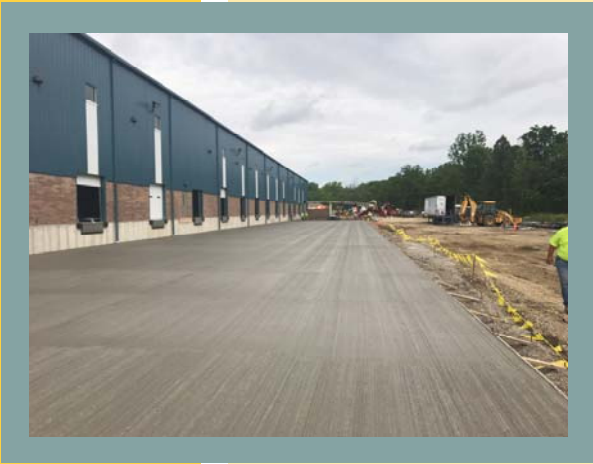
Pic 1: The weather let up, so the dock area concrete has been poured!
