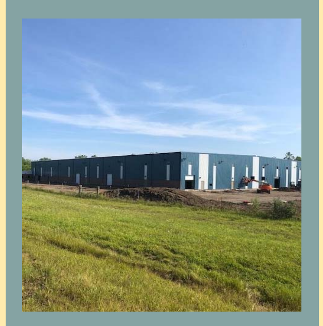
Pic 3: COMTEX II viewed from Highway 250
